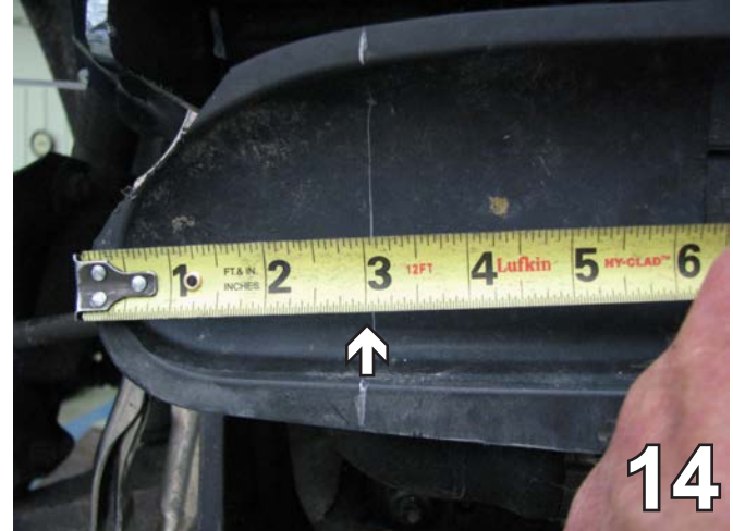
14. On the driver's side, disconnect the temperature sensor. It will need to be relocated. Cut straight down along the edge of the plug plate. On the passenger side, measure 3" over from the end of the frame and cut straight down.
