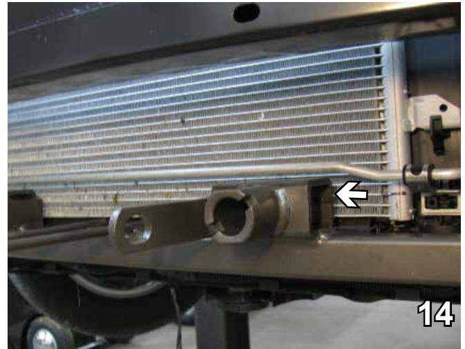
14. There is 1/2" gap between the line and the baseplate.
